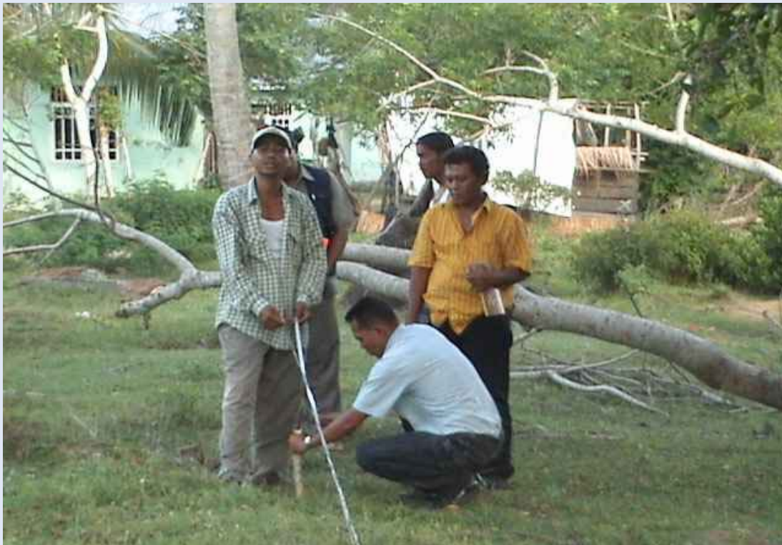
Some men of Kuala Idi Cut village measuring the land before building water tanks.
